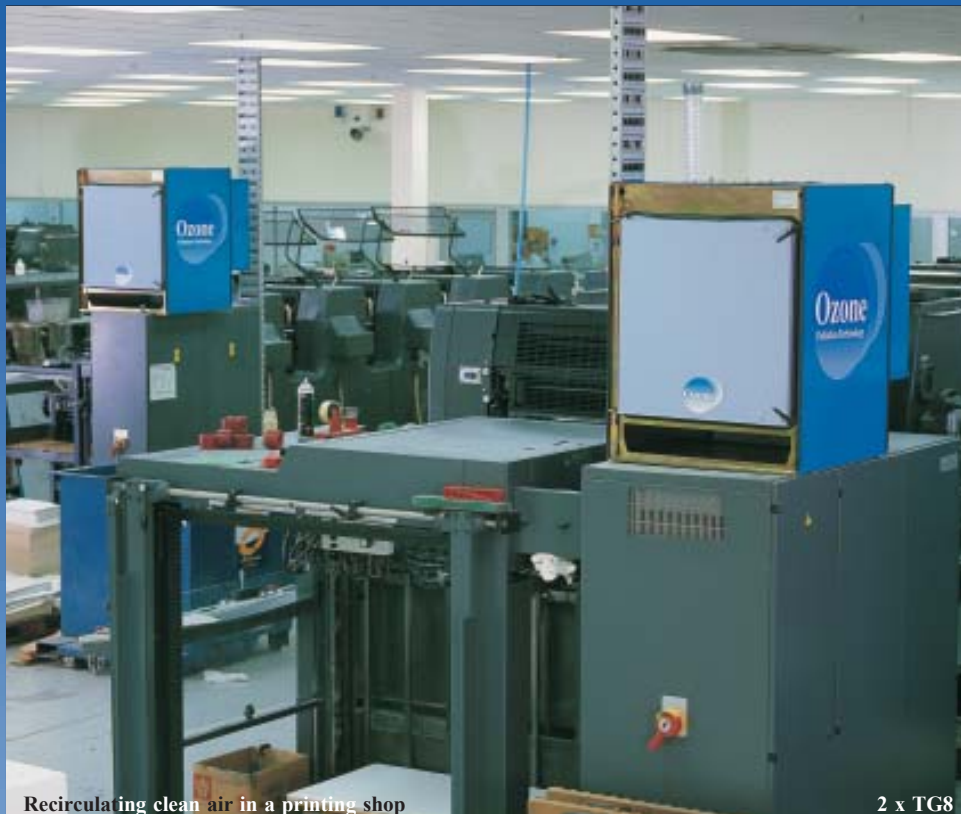
Recirculating clean air in a printing shop
